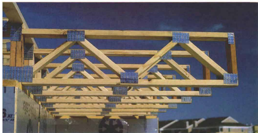
Floor trusses can be cantilevered over longer distances than wood joists. These trusses will support a balcony. Pressure-treated wood was used for the end web as a precaution against rot caused by possible water infiltration. The double vertical web member at the wall provides additional support for the deck loads on the cantilever.
